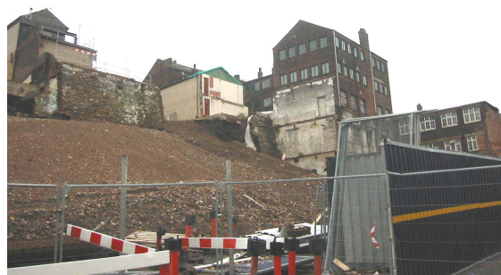
71. Site of the collapsed retaining wall to the rear of Solly Street, viewed from Kenyon Street - Cornhill Works (5) is the dominant building centre-right.
