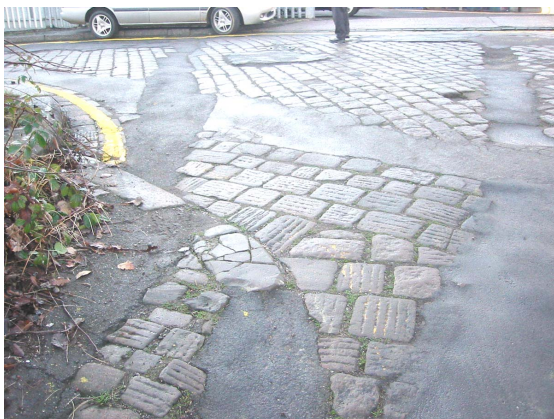
58. Surviving setts in Well Meadow Street - typically laid obliquely to the road line.
