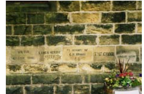
Foundation stones commemorating people who contributed to the building of the Norfolk Hill Methodist Chapel and Sunday School.
