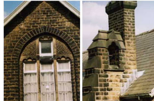
Infants school in Arts-and-Crafts style with herring-bone patterned stonework and large chimneys with angled stone offsets incorporating a belfry.
