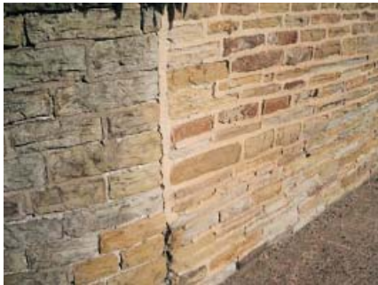
An example (on the right) of unsightly and damaging repointing with hard cement.
