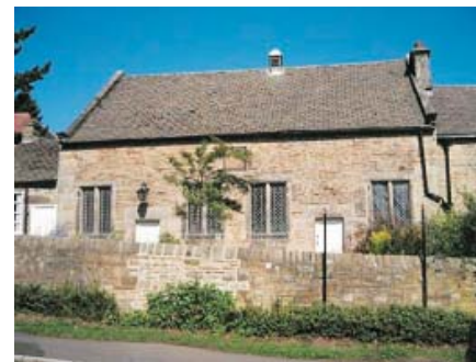
The central section of this wall has been repointed with hard cement mortar.
