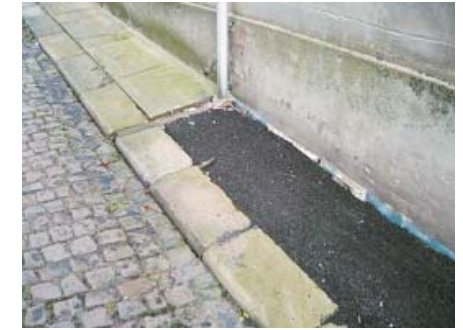
Stone slabs unfortunately replaced with black tarmac.
