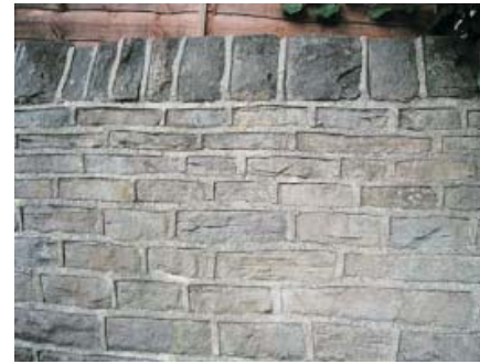
Stone wall badly repointed with hard cement mortar.
