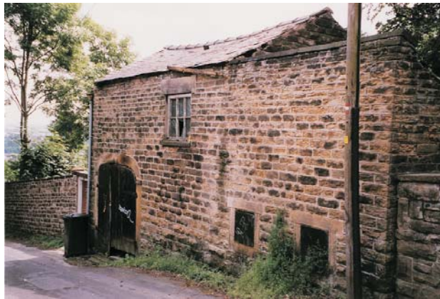
Rear property walls of coursed sandstone backing onto Nos 48 to 54 Birkendale View incorporate stables, carriage sheds and hay lofts.
