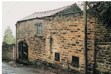
Buildings at risk: graffiti on carriage sheds and stables along Birkendale View.
