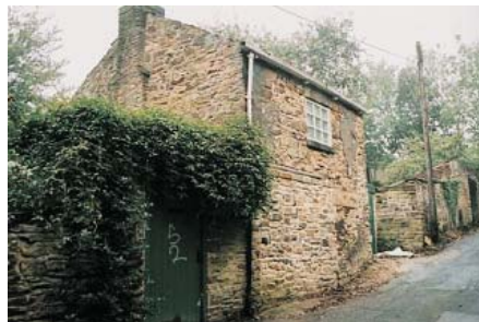
Carriage sheds and stables along Birkendale View threatened by neglect.
