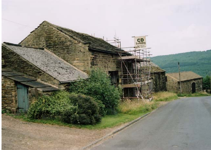
Photograph BHL 18: Buildings at Risk: the eastern gable end wall of this aisled barn at Old Hall Farm collapsed after heavy rain in the winter of 2005. Note too the loss of traditional roofing materials on several of the barns and the replacement of traditional flags with corrugated asbestos and concrete tile.
