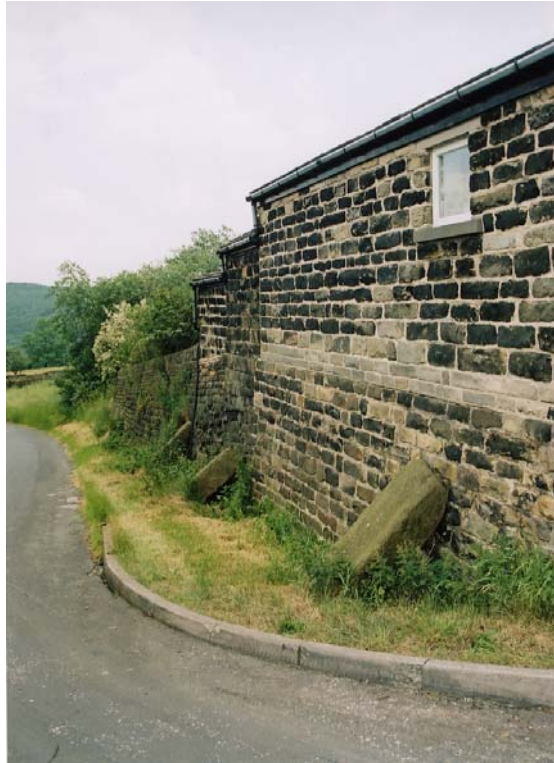
Photograph BHL 14: Rose Cottage is early 19th-century in date and has stoutly buttressed and battered walls. Note, however, the intrusive concrete repointing of the upper walls compared to the original well-disguised and recessed lime mortar pointing of the lower wall.
