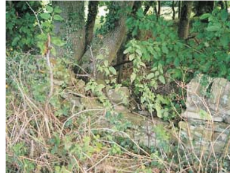
One of the area's characteristic stone walls is damaged by tree growth.
