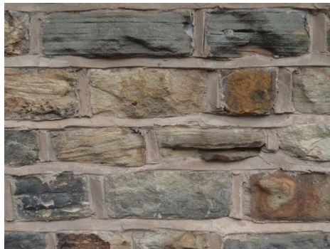
Poor quality 'strap' pointing in cement mortar
