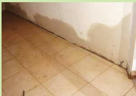
Rising damp shows as a water mark rising up the wall from under the floor.
