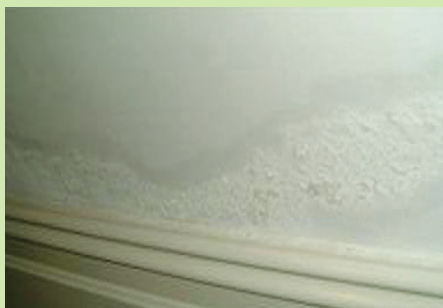
Rising damp is affecting the paint finish causing it to bubble.
