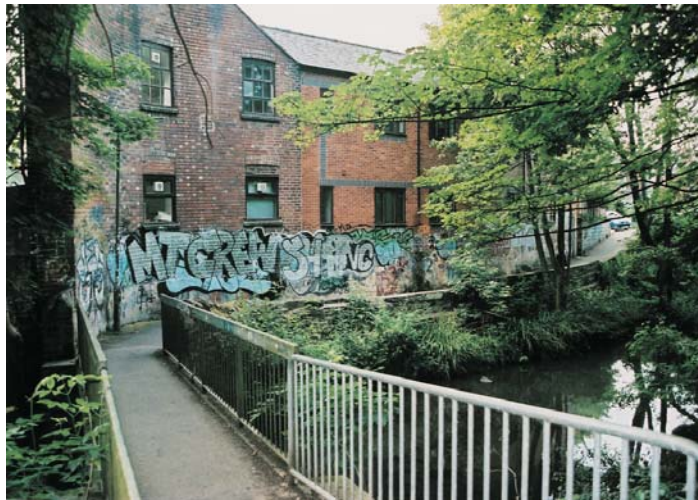
Walls, bridges and railings along the brookside path are marred by graffiti.
