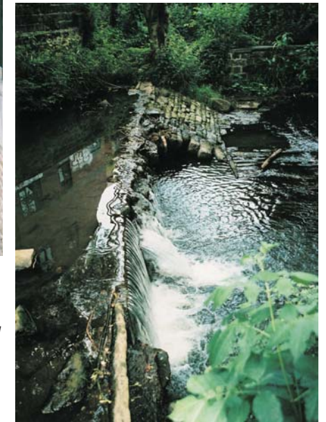
Weirs, rills and cascades along the river bed have deteriorated.
