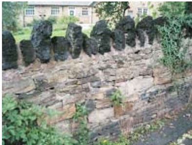
Stone boundary walls are a feature of the area. This one has an unusual coping.
