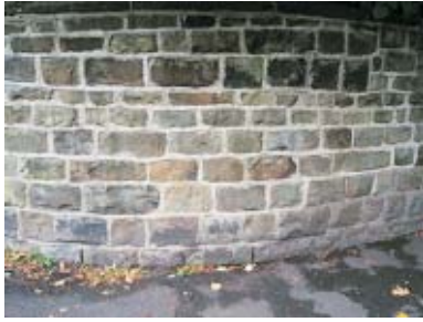
A stone wall inappropriately repointed with hard cement mortar.
