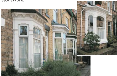
(i) Bay windows altered to Upvc (above). Compare an original timber bay retaining its fine decorative mouldings & sash windows (inset).
