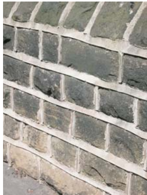
(e) Strap pointing - offensive in appearance and damaging to stonework.
