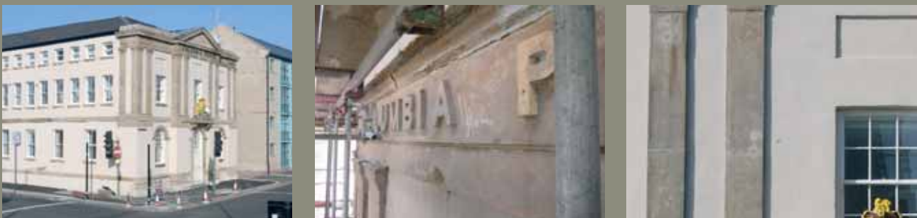
Figure 20: Columbia Place after restoration of external elevations and picture of the detailed work being undertaken
