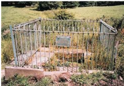
The well basin is damaged and patched with concrete blocks.
