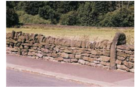
Badly repaired walls.
