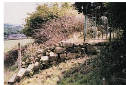
Broken steps leading to the well.
