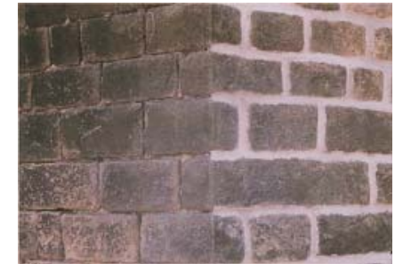
Same building – two different mortars: original lime-based mortar on the left; cement based repointing on the right.
