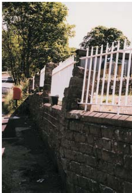
Broken walls and railings and abandoned temporary classrooms at The Old School.
