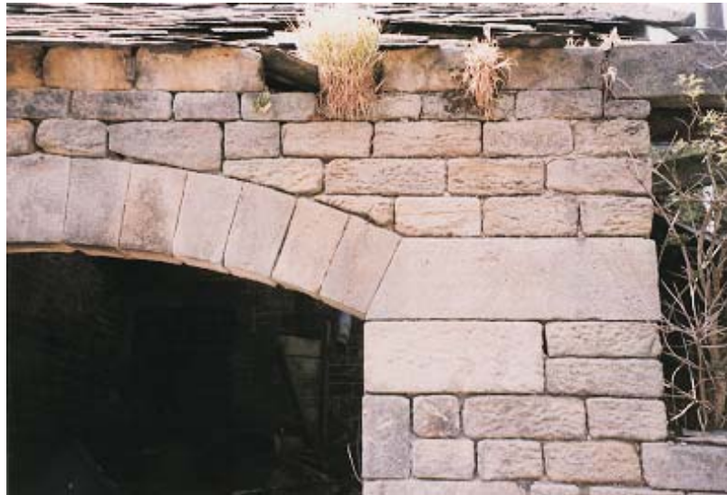
The barn opposite St James's church, showing the construction of the cart shed lintel and the adjacent window or pitching hole.
