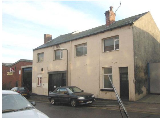
97. 84-90 Randall Street (11) - the brickwork is now rendered over and the windows replaced inappropriately.
