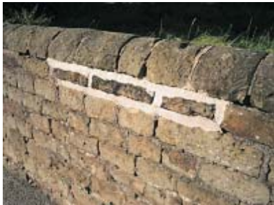
Example of unsightly and damaging re-pointing of natural stone wall.
