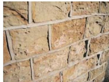
'Ribbon pointing' spoils the appearance of a traditional stone wall.
