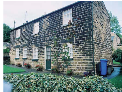
Broken or collapsed boundary walls where the conservation area adjoins Wheata Wood.
