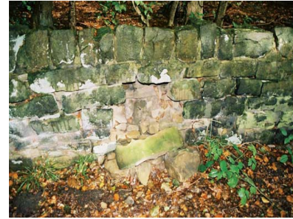
Broken or collapsed boundary walls where the conservation area adjoins Wheata Wood.
