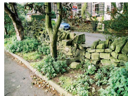
Broken walls that have not been repaired to the same standard as the original.
