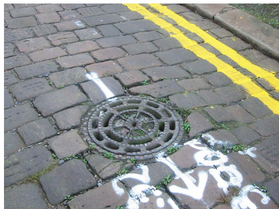
28. Cast iron wheel-pattern drain-gratings survive in the carriageway along Cupola, surrounded by original sets.
