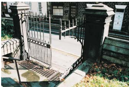
One of the main gates' posts is broken.
