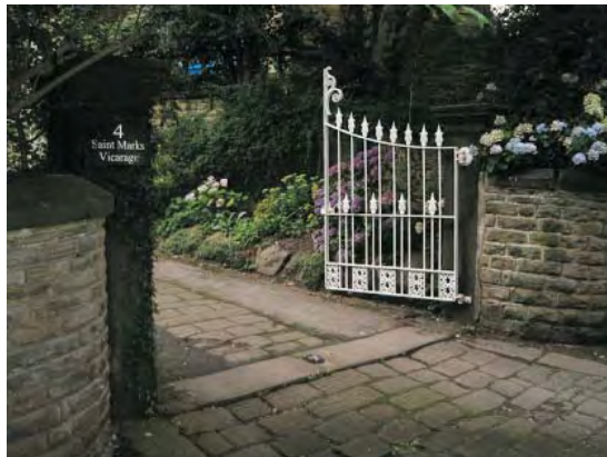
Stone gate piers and stone setts at entrance to St. Mark's Vicarage
