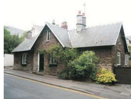
Former lodge in Park Lane. Note the poor quality repointing at the lower right hand side of the facade.
