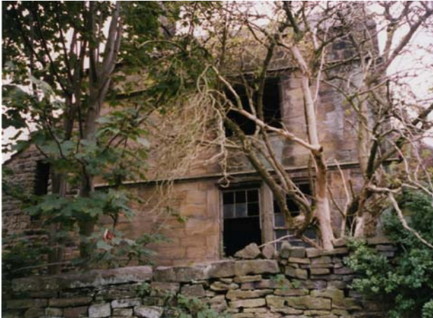
Poor state of repair of Old Hall Farm.
