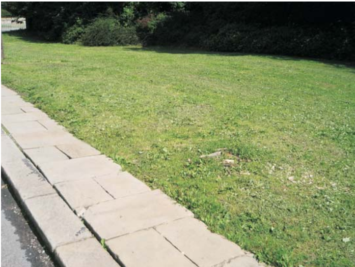
Natural stone paving and grassed area at south end of Beauchief Abbey Lane
