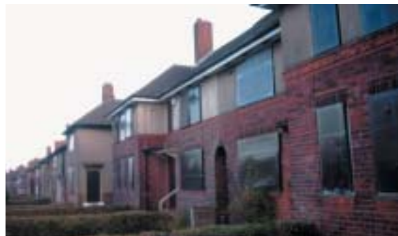
3. Housing to be replaced
