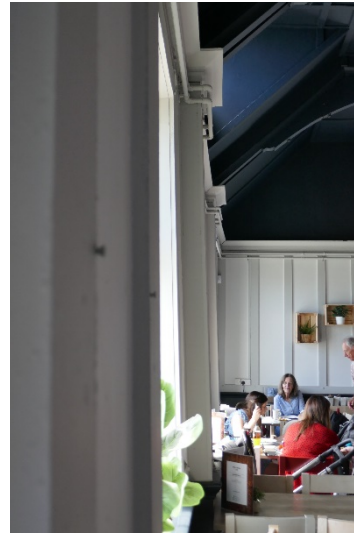
Photo showing front elevation leaning out internally, against vertical in background
