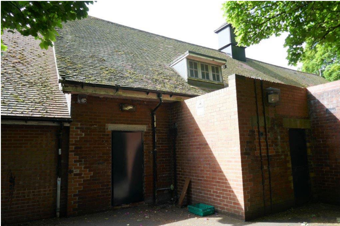
Photo 3 – Roof sag rear elevation and Dormer Window backwards lean.
