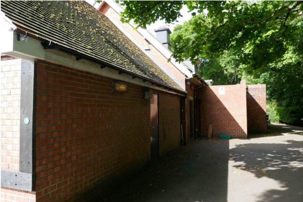
Photo 7 – Missing gutter section rear elevation toilet block.
