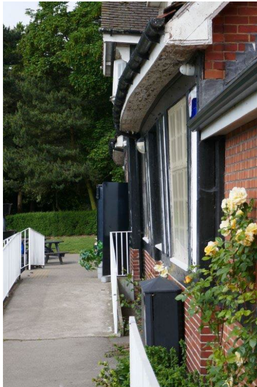
Photo 1 – Bulging of soffit beam and forwards movement of front elevation.
