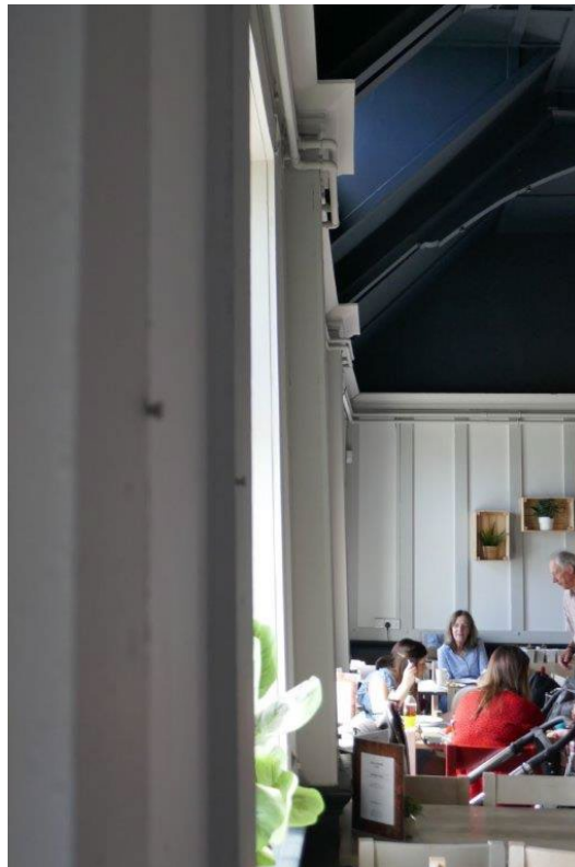
Photo 8 – Outwards lean to front elevation window frames.
