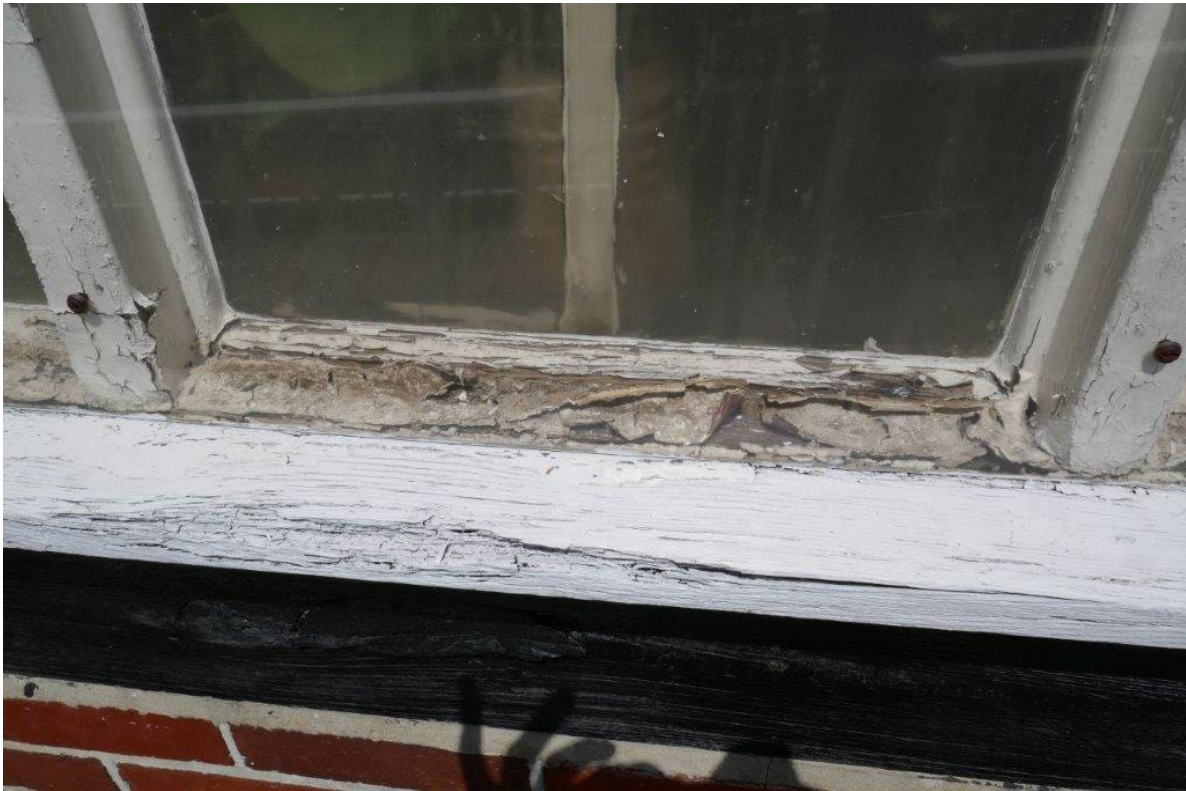
Photo 9 – Rotten window frames exacerbated by fixing of Perspex to front.
