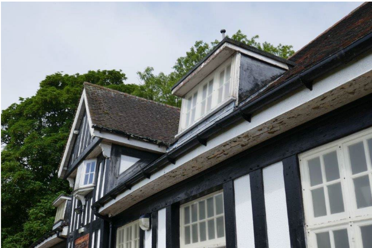
Photo 4 – Backwards lean to Dormer windows Front Elevation.
