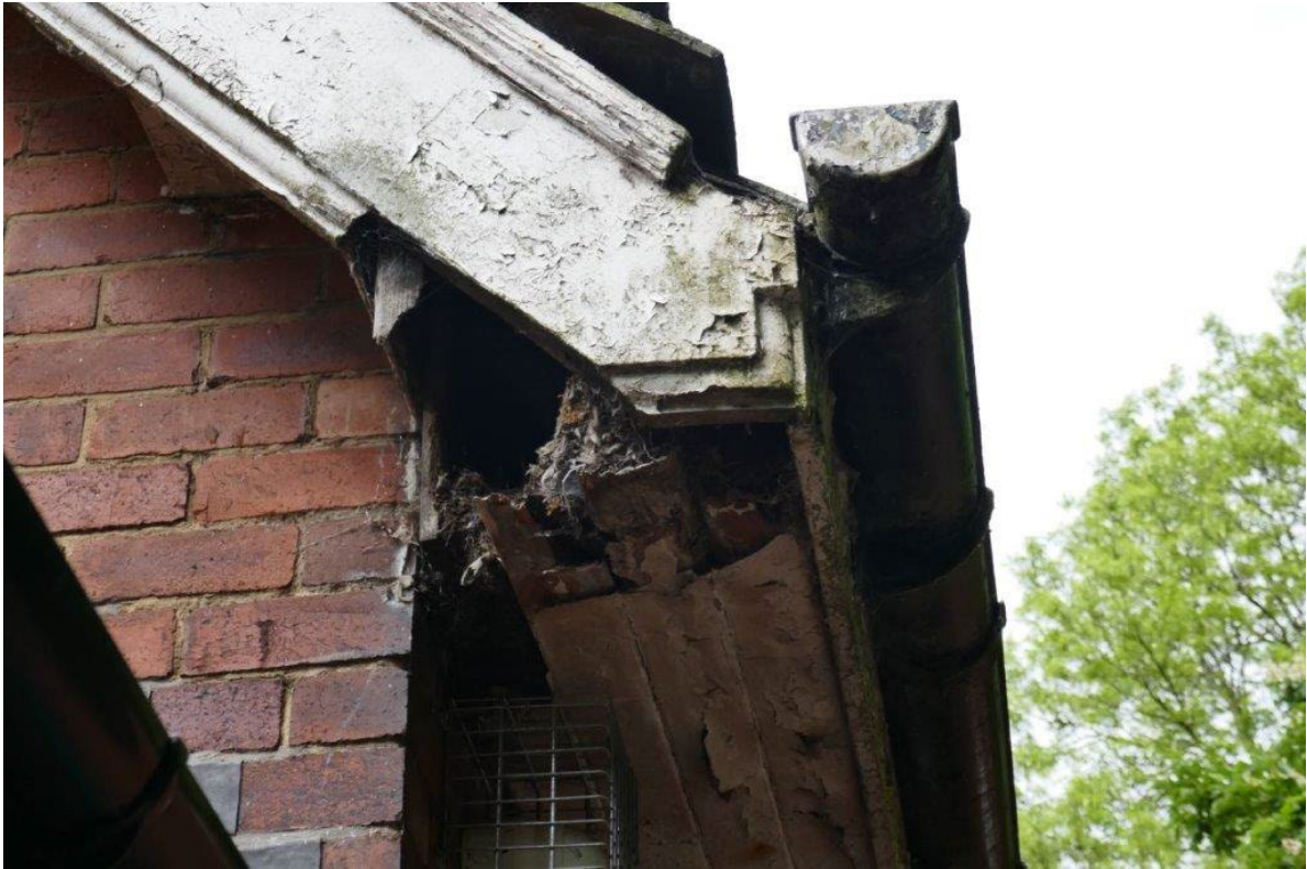
Photo 5 – Bird entry/missing soffit rear elevation.
