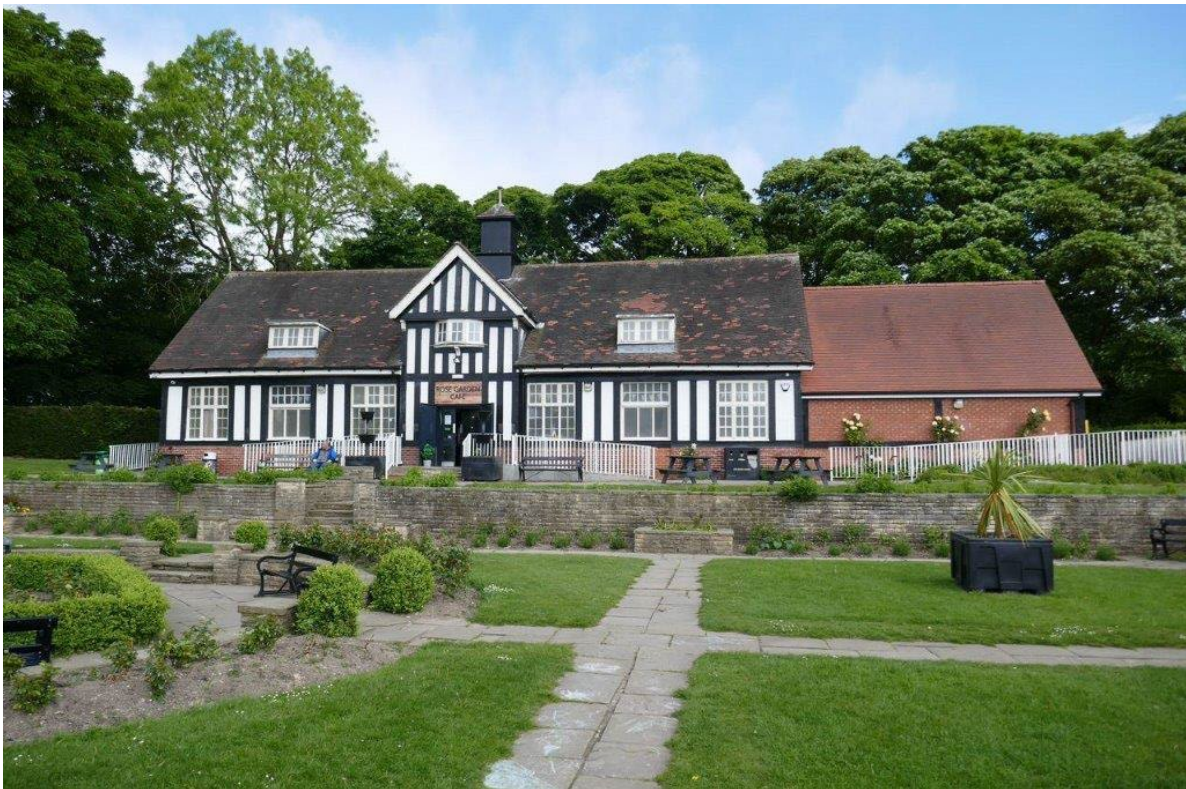
Photo 2 – Roof sag front elevation.
