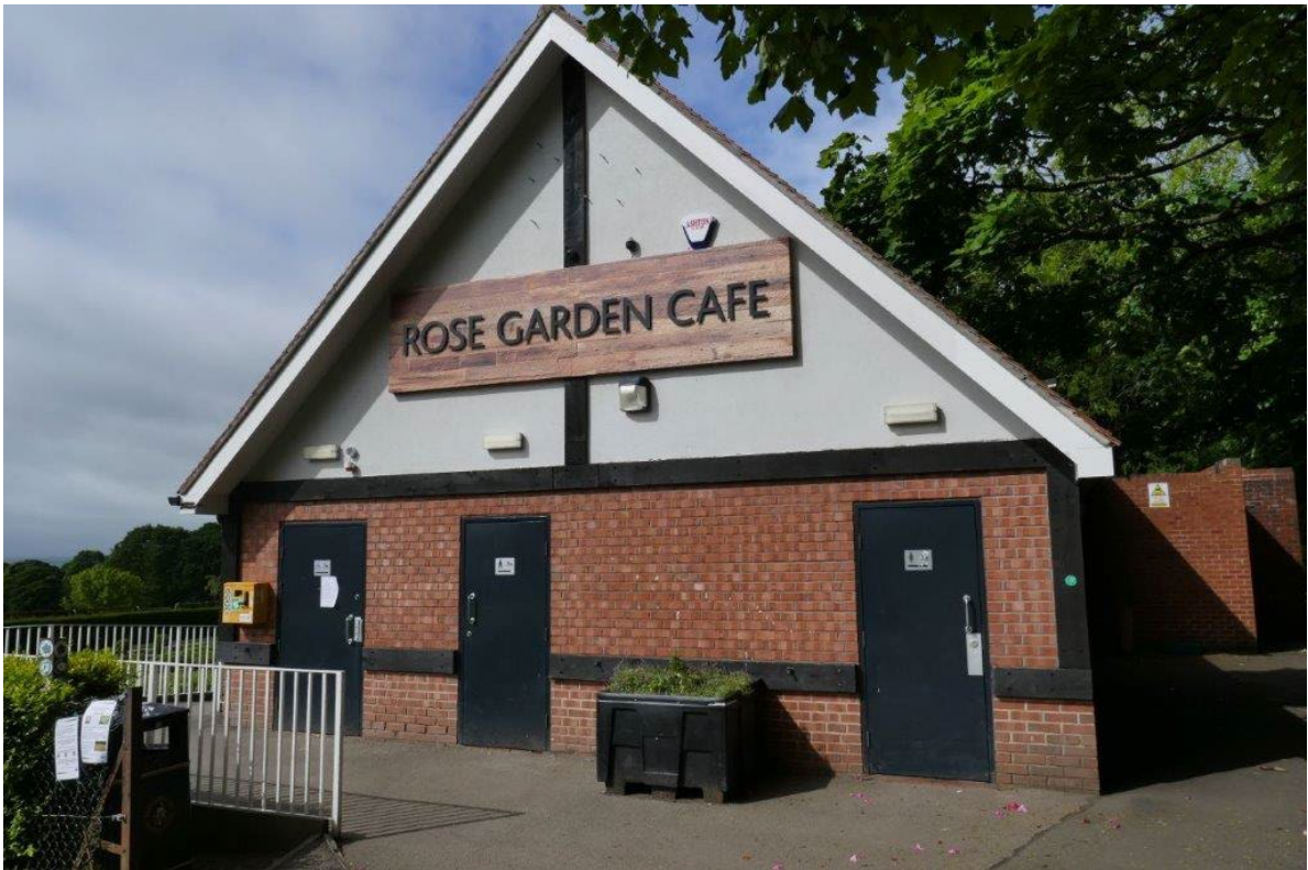
Photo 6 – Poor detailing box end/soffit beam toilet block extension (LHS photo).
