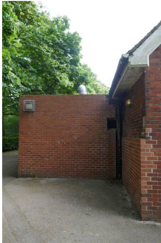
Photo 11 - External skins of brickwork added at a later stage. Extends ½ wall on RHS covering an outside urinal.
